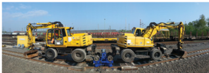
Figure 1: Shaker (blue) with two excavators on a straight track, picture distorted by a photography effect (Picture: Ingenieurbüro Dr. Heiland)
