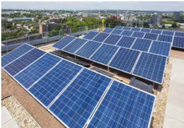
© John Sturrock Solar panels on the roof of Five Pancras Square, King's Cross
